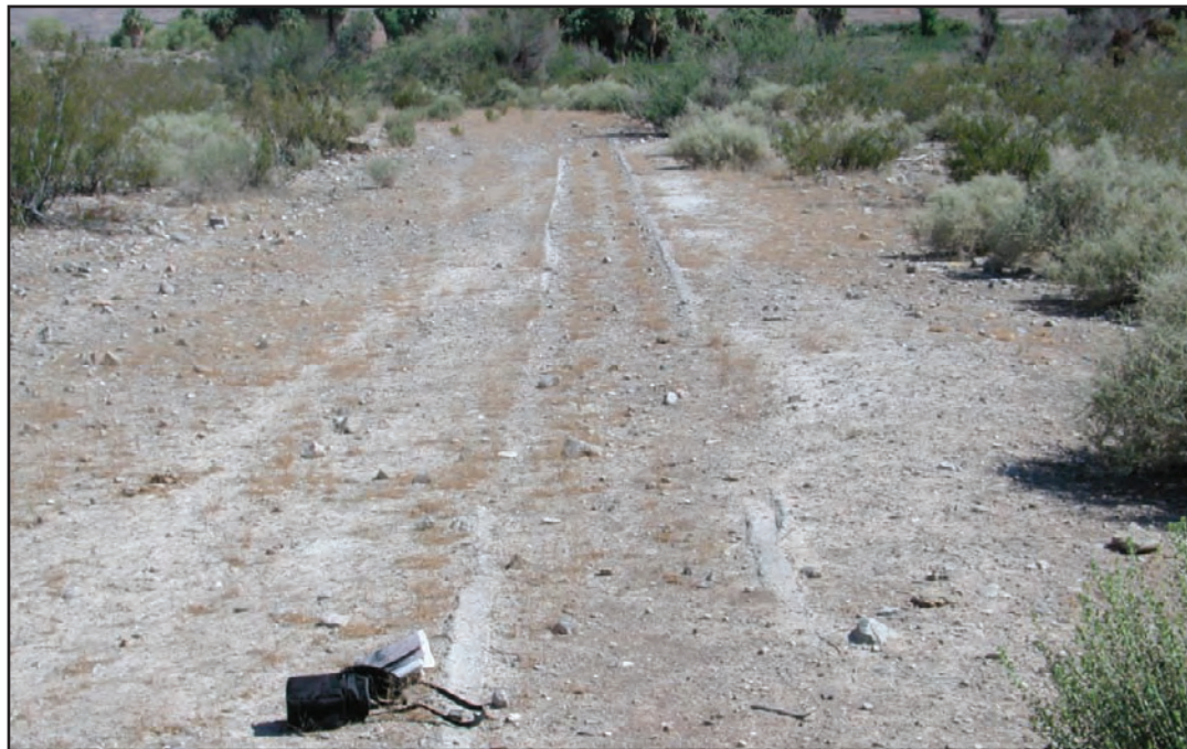
B. Former concrete irrigation ditch south of Cardy Lamb Swimming Pond that has been completely filled in with dirt.
