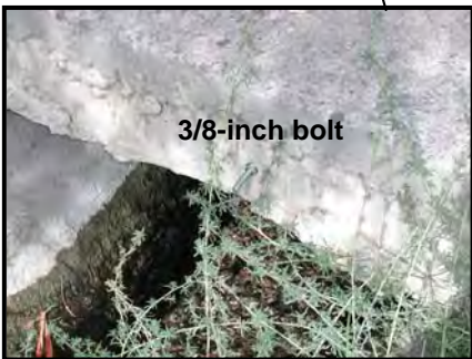
3/8-inch bolt RP-1 (1,798.38 ft) (Tape down point to measure water level)
