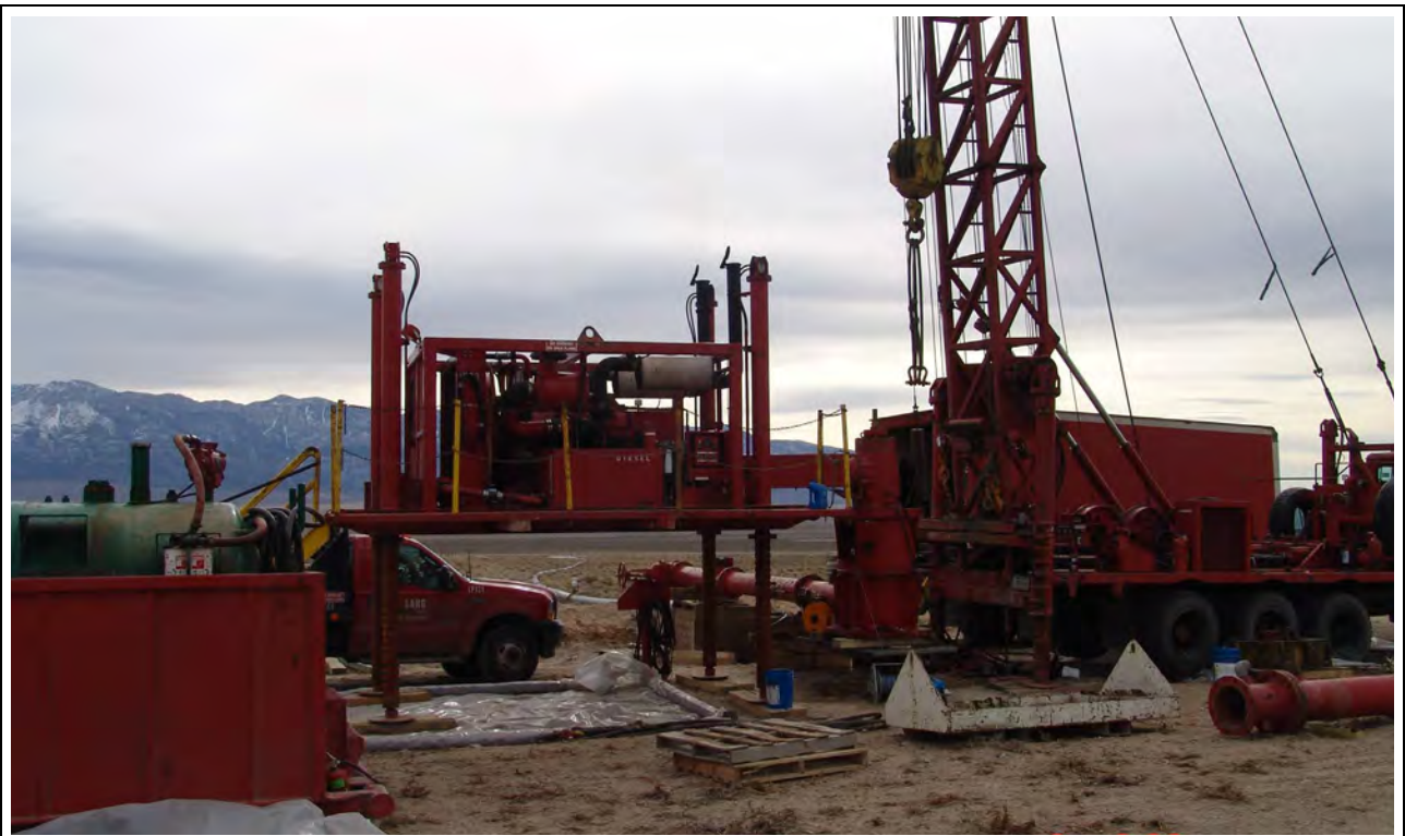
Figure A-3 184W105 Test Wellhead Equipment with Generator
