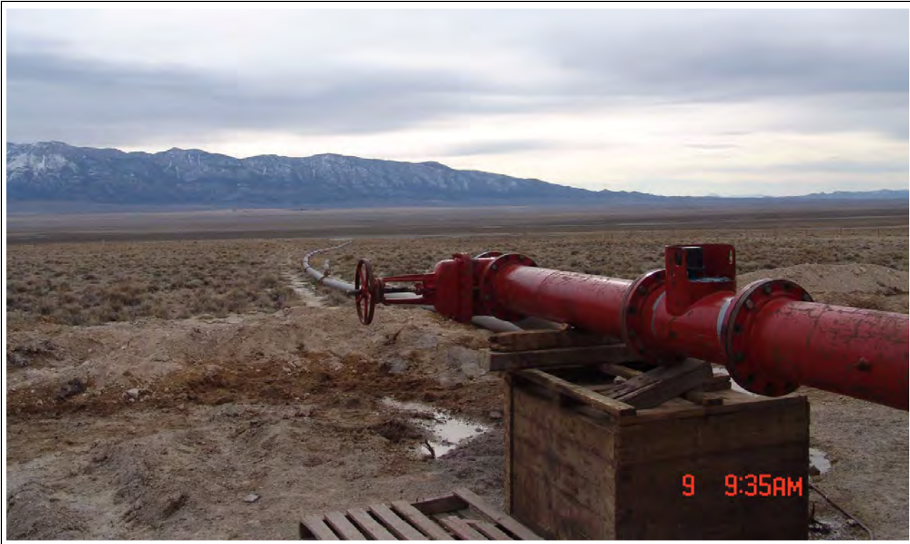
Figure A-4 Discharge Piping, Facing East from Well Site 184W105
