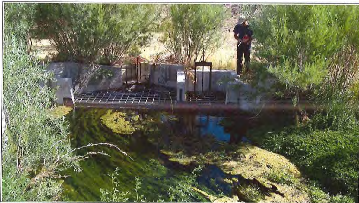
Figure 3-55 View Looking Downstream at the Lund Irrigation Company's Diversion Structure on Lund Spring
