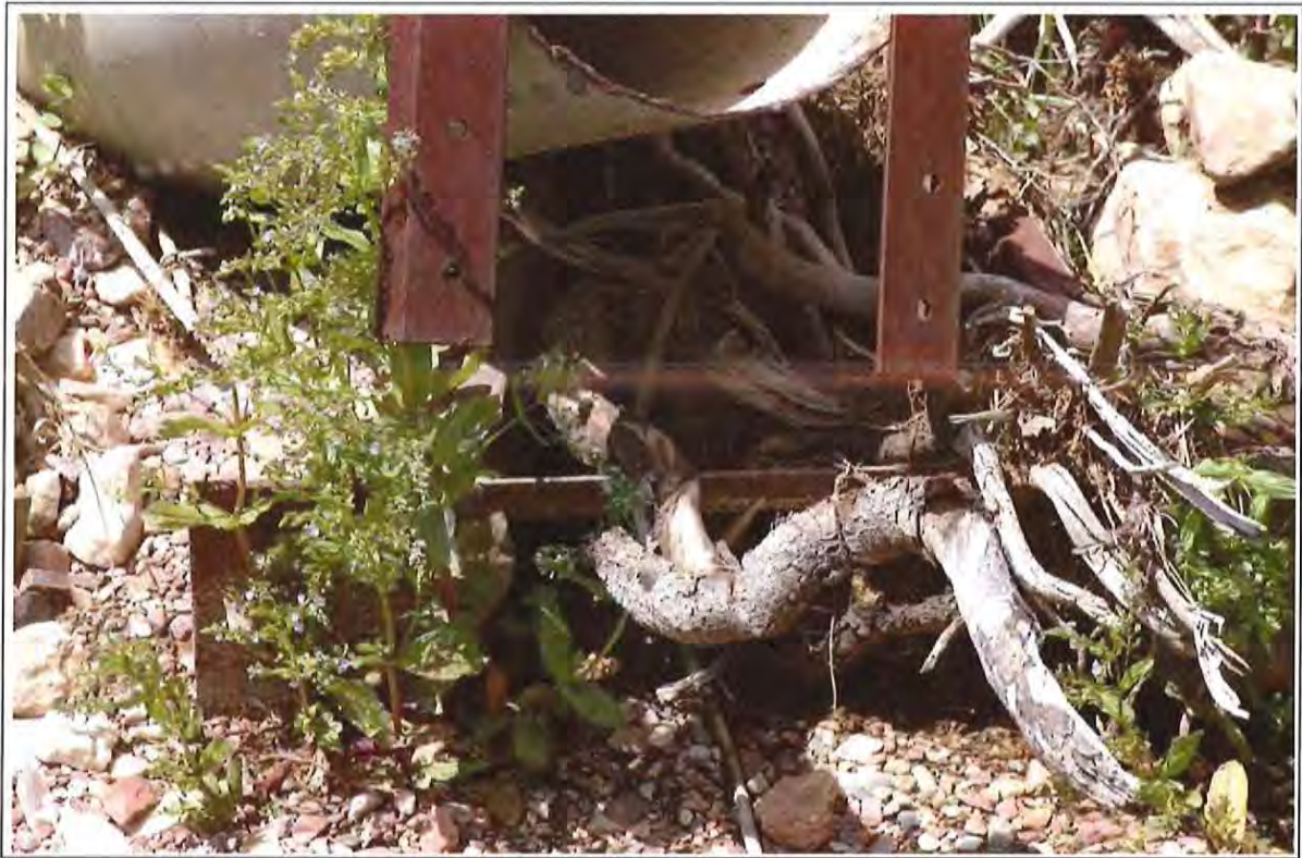
Figure 3-108 Partially Buried 6-in. Parshall Flume Found in Channel below Geyser Spring Lake Valley, Nevada
