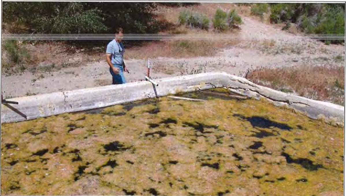
Figure 3-83 Stock Tank and Diversion Pipe at Coyote Spring, Dry Lake Valley, Nevada
