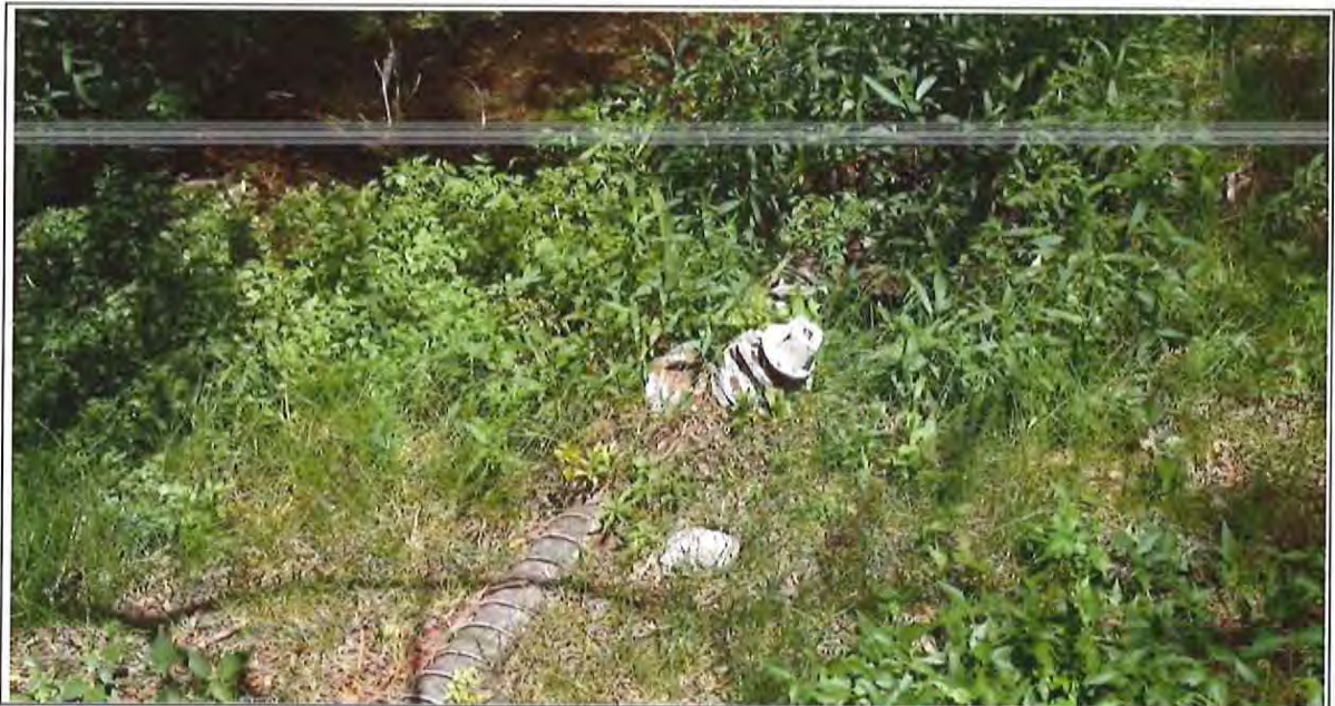
Figure 3-30 Gate Valve and an Exposed Section of Redwood Pipe along Southern Channel Diversion of Swallow Springs
