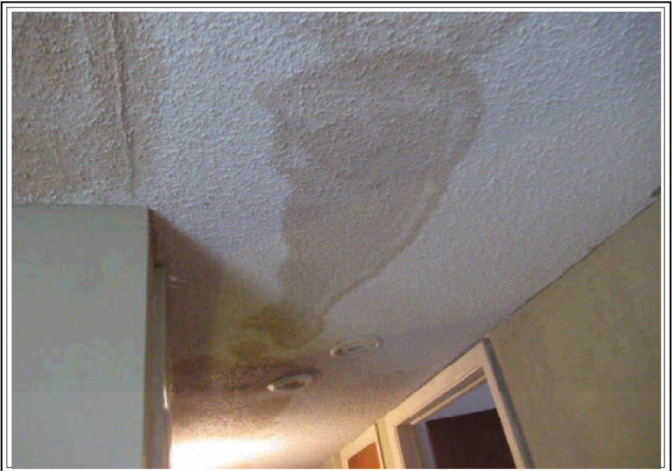
Comment: Water damage from faulty roof.
