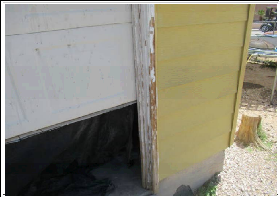
Comment: Exterior paint-peeled and cracked
