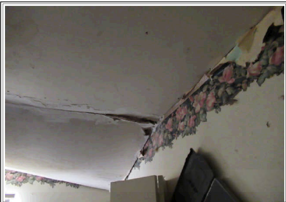
Comment: Collapsed ceiling from faulty roof/water damage.
