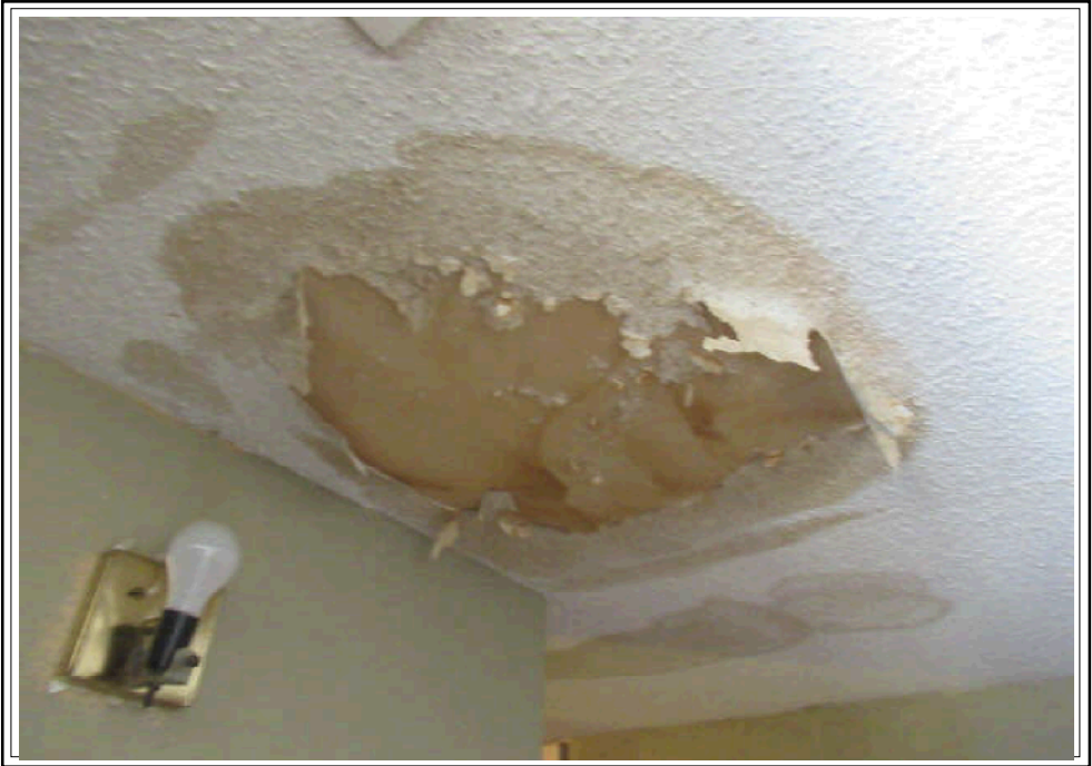
Comment: Water damage from faulty roof.
