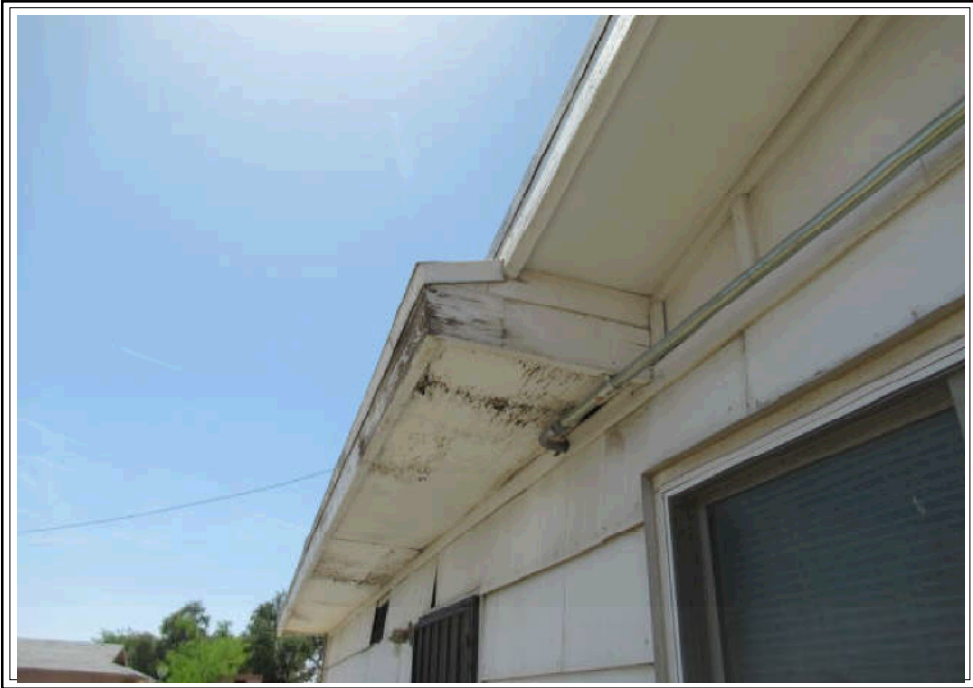
Comment: Exterior paint-peeled and cracked
