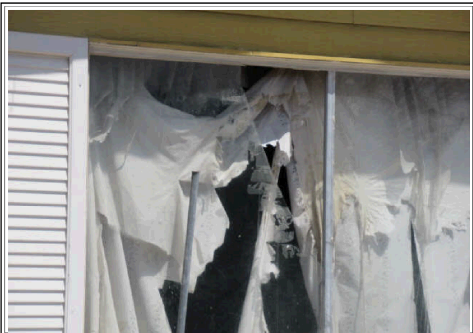
Comment: Broken window
