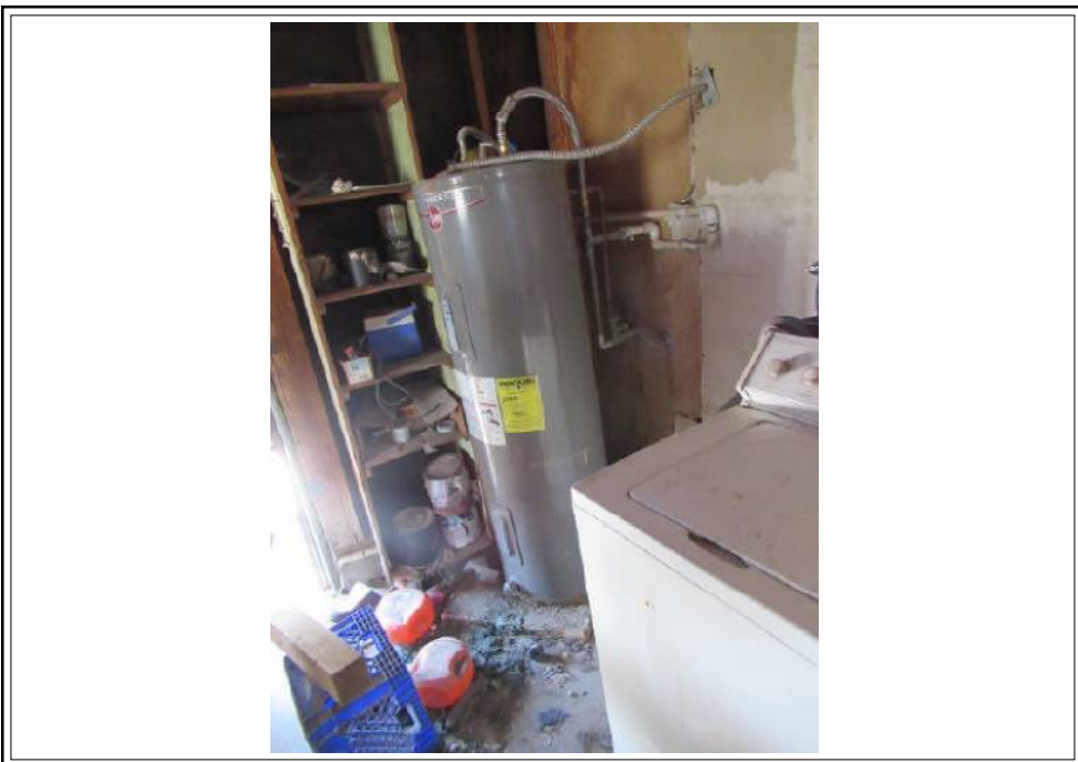
Comment: Water heater
