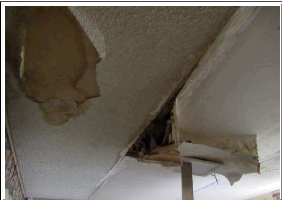
Comment: Collapsed ceiling from faulty roof/water damage.
