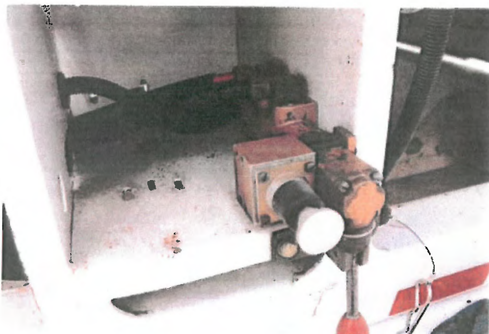
Figure 5-14. Dump Control Valve – Unit #6775
